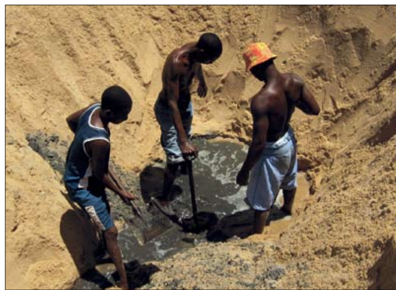
Knee deep: Unblocking Beira's sewers has required the skills of a nation well acquainted with the problem — Italy, whose sewers were once regarded as the 'most compromised anywhere'
